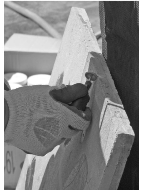
Fig. 8. Routing a crack in a panel as part of cementitious patch repair, 2010.
