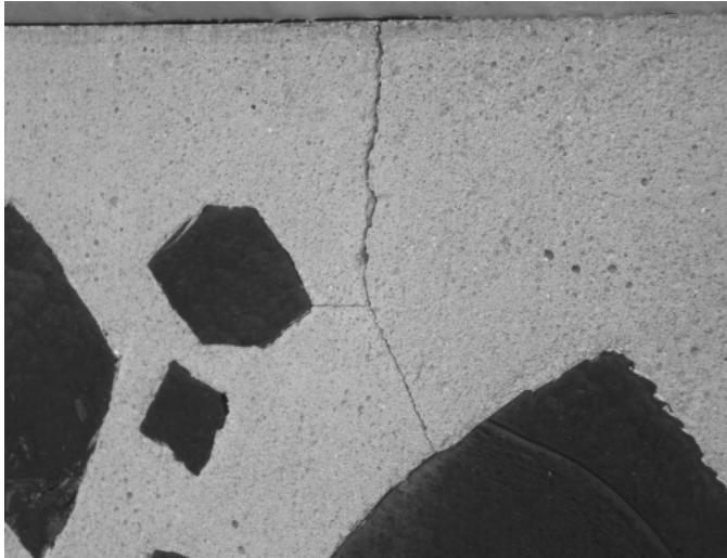
Fig. 6. Typical crack in a dalle-de-verre panel, stretching from glass to the edge of the panel, 2009.
