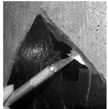
Fig. 5. Translucent coating degrading on interior dalle-de-verre panel, 2009.
