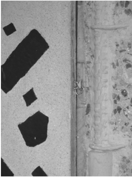
Fig. 4. Attachment of dalle-de-verre panel to cast-in-place concrete, 2010. The concrete on the left side of the image was demolished, and the steel reinforcement was cleaned and coated with a rust-inhibitive coating in preparation for patching.
